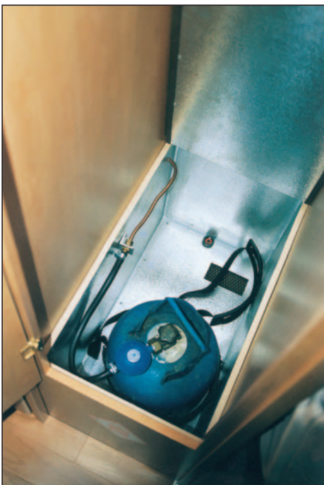
...gas cylinder locker.
