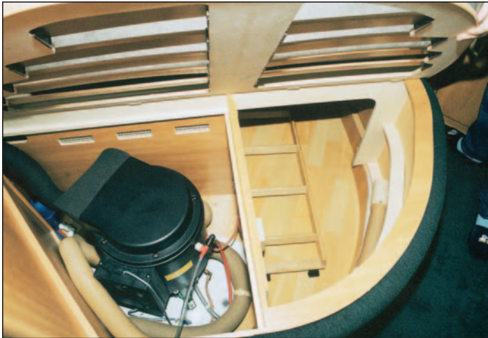
Lift-up the end of the bed base for access to locker and powerful Truma Combi water/space heater.
