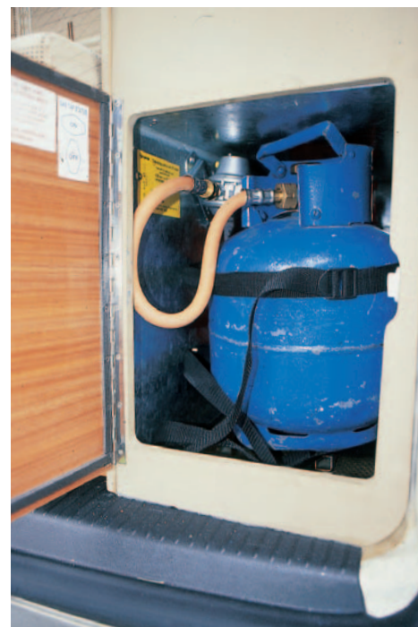
The entrance to the gas locker was barely wide enough to get a cylinder out. Auto-Sleepers, I was told, has addressed this problem.
