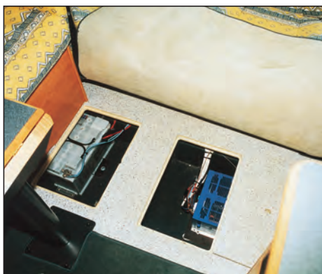
Roll back the carpet to find trapdoor access to the auxiliary battery and charger. More hatches enable water tank cleaning.
