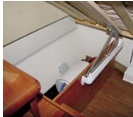
The water heater is small - just five litres
