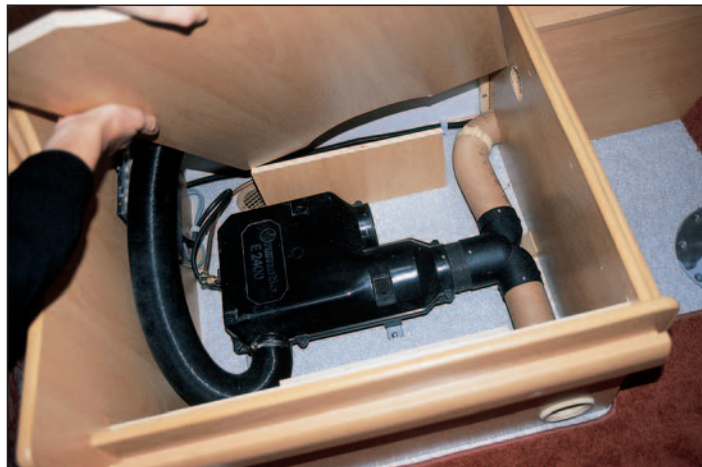
The gas-fired Truma blown-air heater is under the forward-facing dinette seat.
