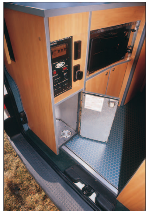
The electrical control panel deals with both mains and 12V circuits and is housed - along with the single cylinder gas locker - in the base of the kitchen unit.
